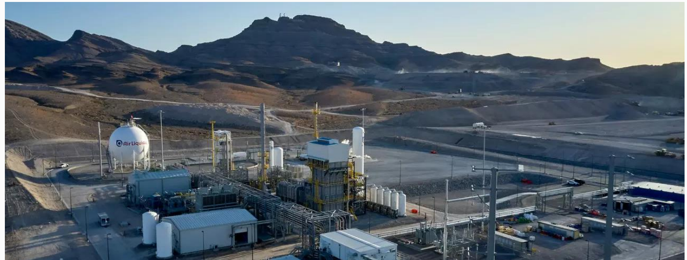
Steam methane reforming and liquid storage facility - Air Liquide - Apex, NV
